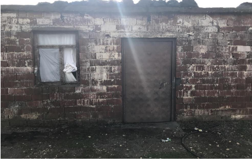
The damaged frontage of a house in Çakirtutmaz after raids.
